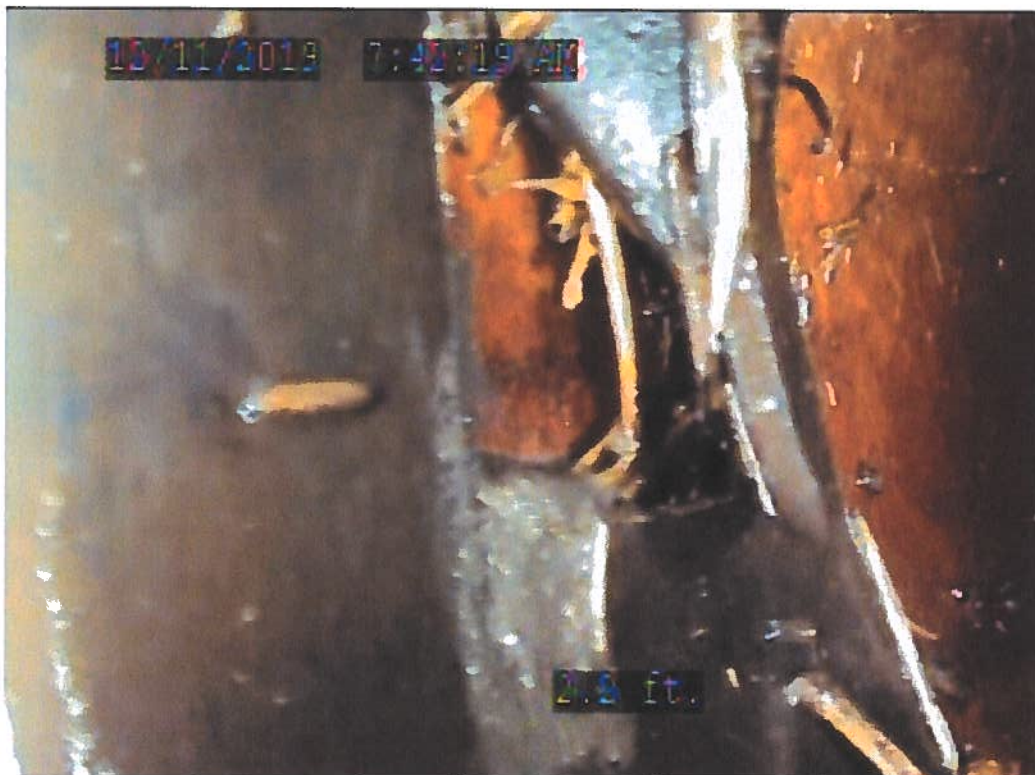
Figure 13: Single wall HDPE to VCP. Joint misshapen.
