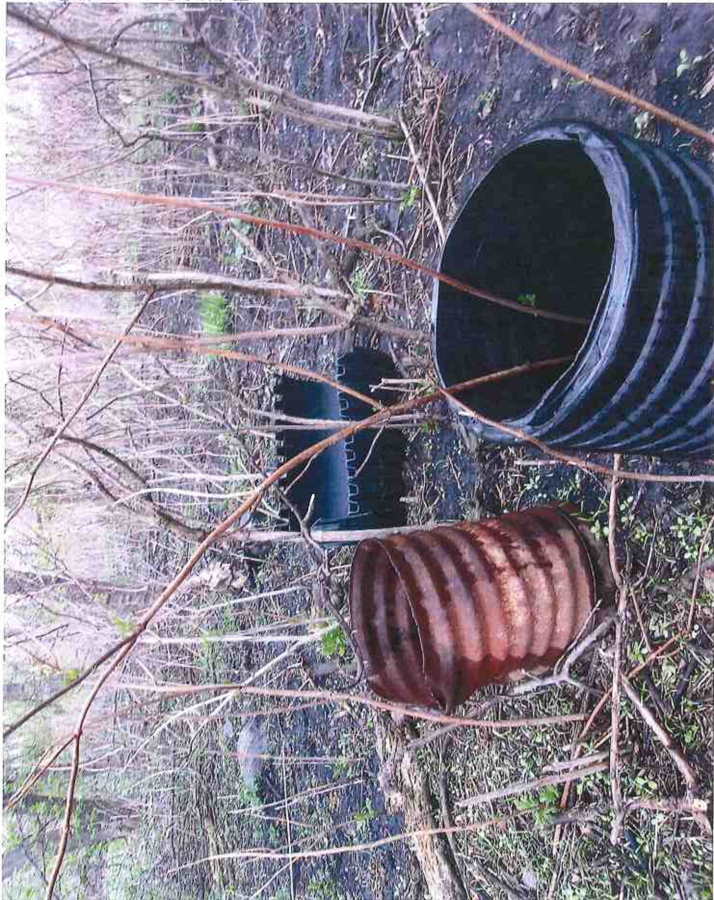
TILE REPAIR PIECES DISCARDED
