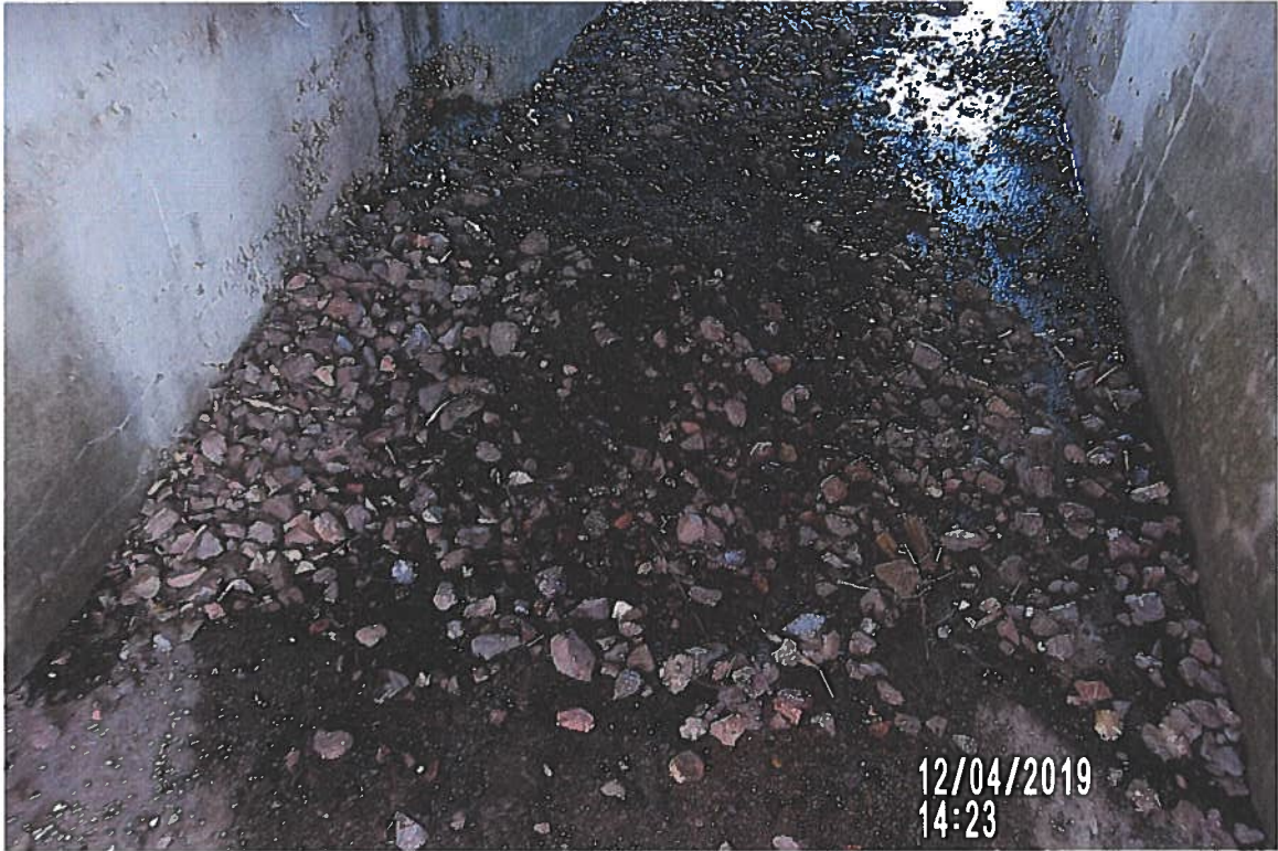
PICTURE BALLAST ROCK FALLING IN BOX CULVERT # 2460
